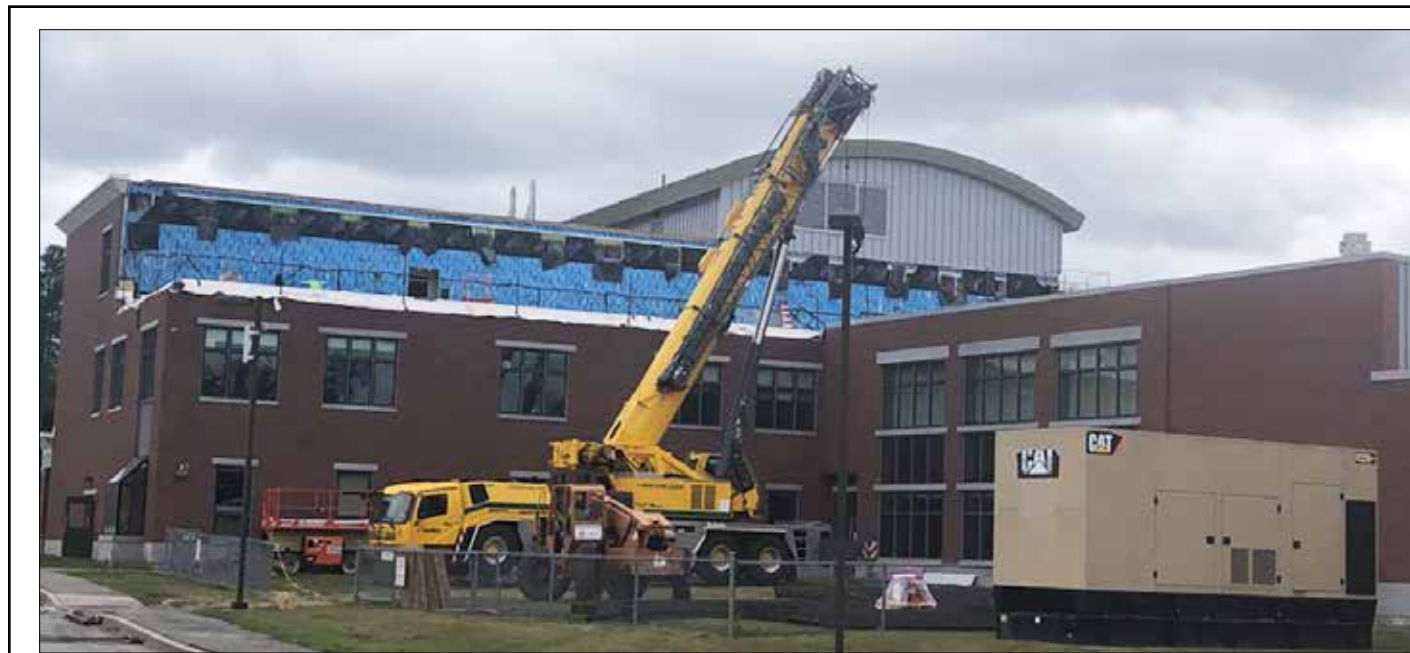
CONSTRUCTION WORK IS ON SCHEDULE for the 3rd floor build-out at Hampden Academy, according to Director of Facilities Bill Booth. The crane arrived on site August 10, and the steel was lifted into position after about a week. The next items needed are the windows, which have been delayed—not because of the steel framing but because of the glass. Mr. Booth said he still expected the project to be completed by April. He said there should be minimal disruption to the students. There may be some background noise when the construction crews install the framing and shoot it down into the concrete deck. Also, the third floor corridor will be partitioned to ensure that the construction workers can get up to the project area, and the stairwell closest to the football field will be off limits except for emergency egress.
